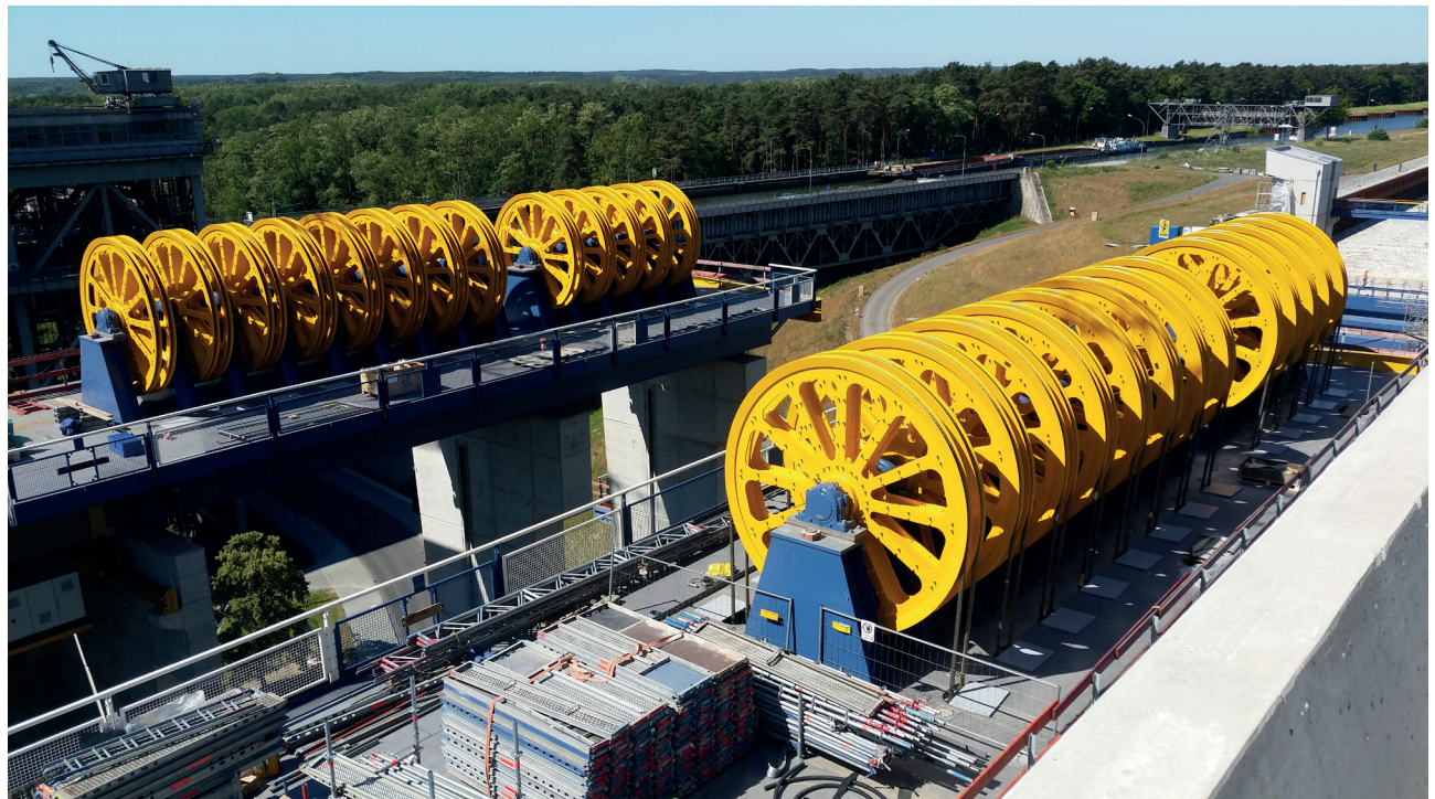
View of a part of the total of 112 installed double cable pulleys. In the background left the old ship lift.
