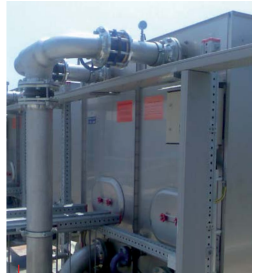
Wet cooling tower on roof
