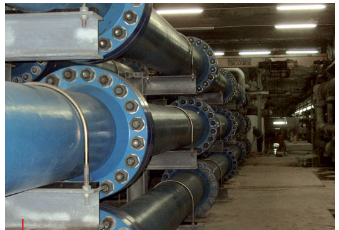
Three-chamber pipe feeder system (P.E.S.), level -2,400 m
