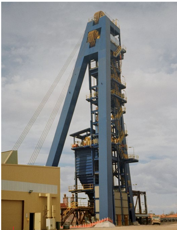
Headframe with hanging guide frame
