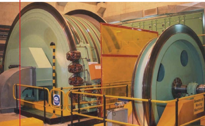
6-Rope Service Winder and 2-Rope Auxiliary Winder
