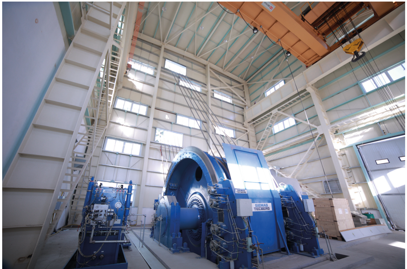
Fig. 1: Already in operation - the 6-rope Koepe hoisting machine of the service shaft.
