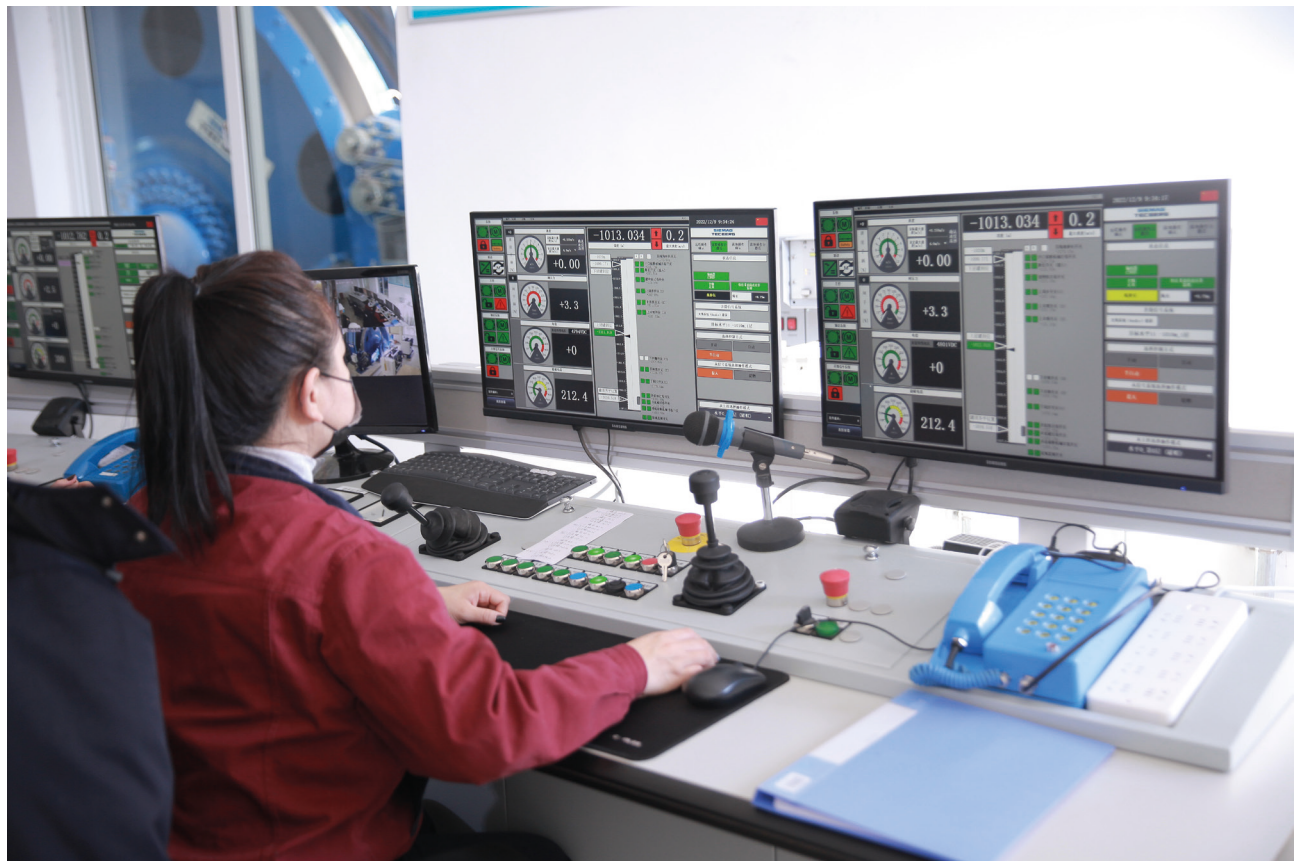
Fig. 3: The special feature of the three hoisting systems is the central control system. The control room is located in the hall of the hoisting machine of the service shaft. In normal operation the hoisting systems in the production and service shaft are all in automatic lifting operation. Furthermore, the two systems in the service shaft are fitted with wireless communication devices that enable the hoisting equipment to be controlled from the cage direct. This enables personnel to reach different levels direct.
