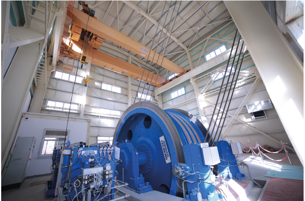
Fig. 2: Also already in operation - the 4-rope Koepe hoisting machine of the service shaft.
